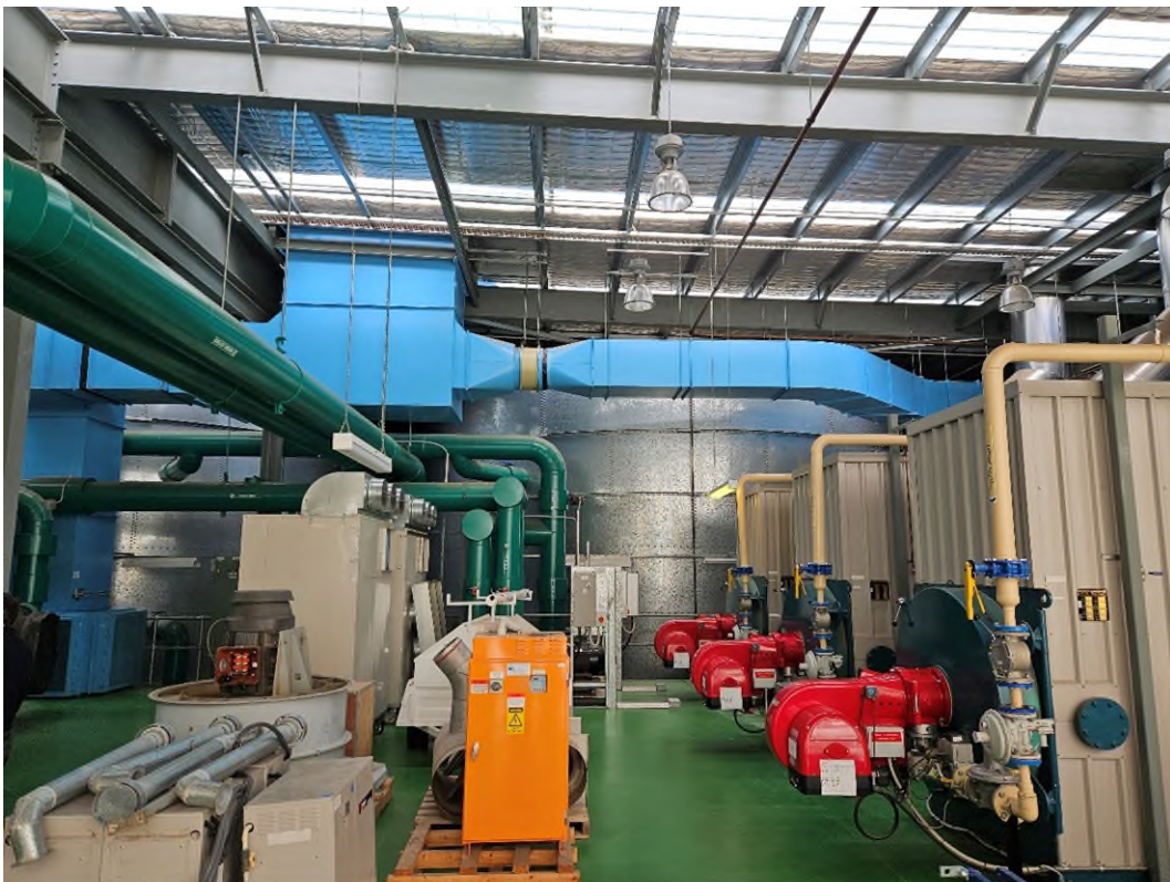
Figure 4 Example of water tank - Building Services Building – 45A
