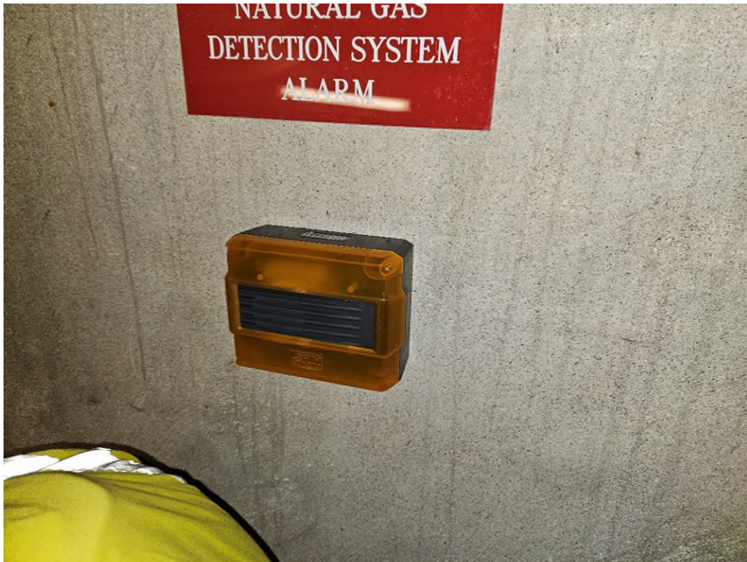
Figure 3: Natural gas detection alarm
