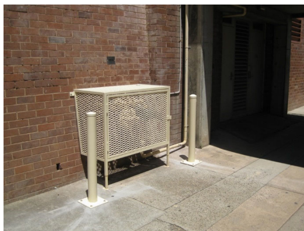
Figure.1: Typical ANU gas meter enclosure
