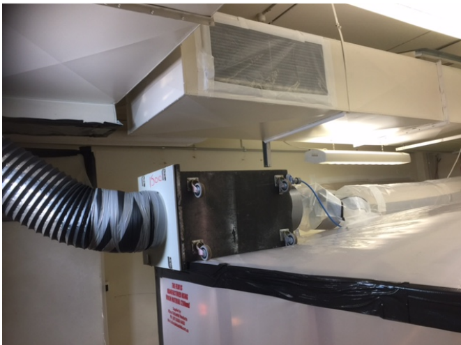
Negative pressure unit to draw in cool air for laser equipment
