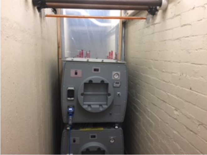
Negative pressure unit
